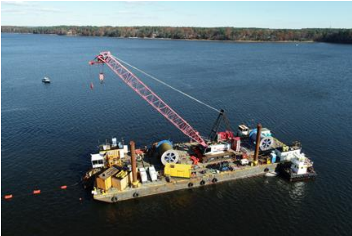
Photo 16. Cable 3, Flight 9, 11/06/2019. Cable lay barge in channel winching jet plow to it. Blue spool holds cable. Note cable coming off barge on the left of the photo, supported by orange floats.
