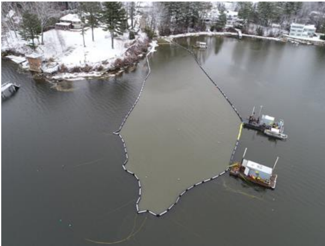
Photo 46. Hand Jet, Flight 1, 12/11/2019. Cable burial using two divers in turbidity barrier on east side.
