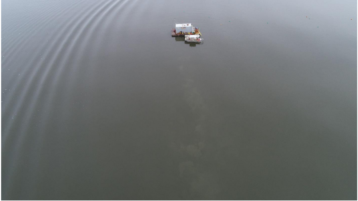
Photo 33. Hand Jet, Flight 2, 11/12/2019. Diver burial in channel with dive support barge and faint turbidity plume.
