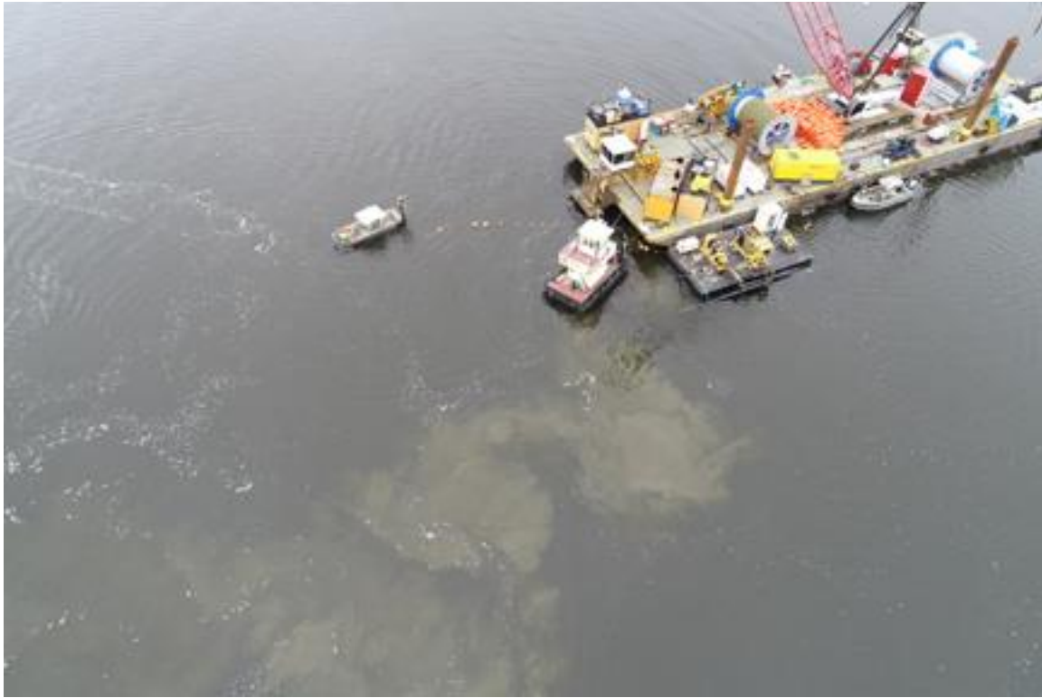
Photo 30. Cable 3, Flight 12, 11/07/2019. Turbidity plume off stern of lay barge during completion of jet plowing.
