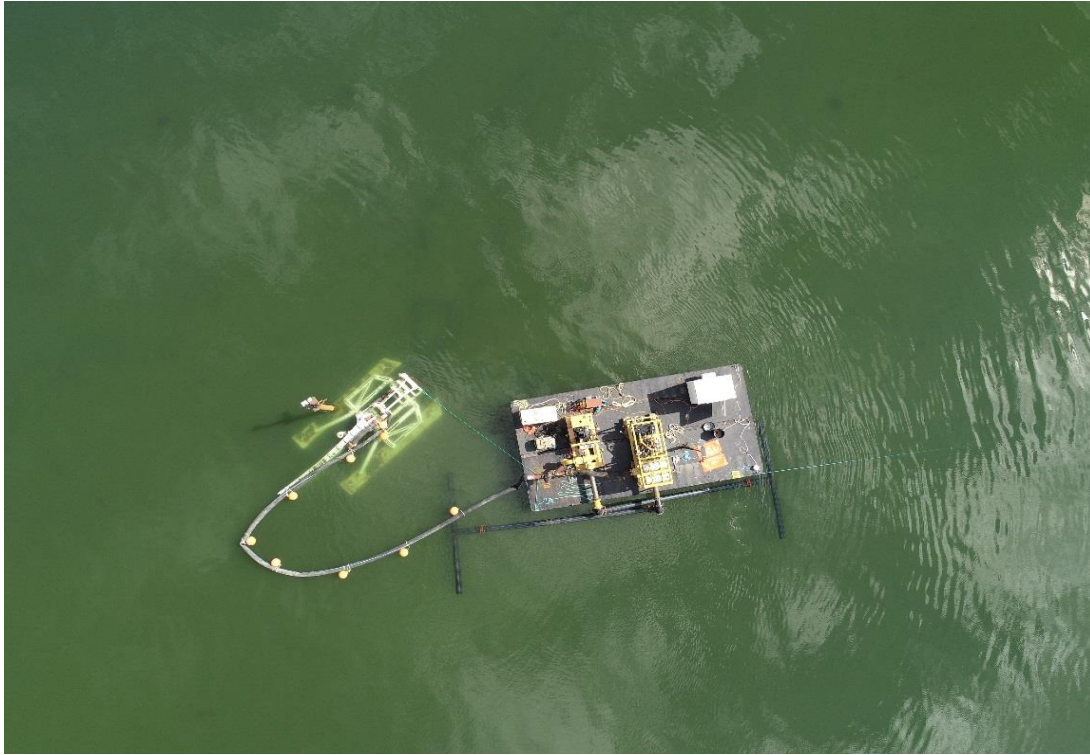
Photo 1. Jet Plow Trial, Flight 1, 9/9/2019. Stationary jet plow in position with pump barge, in position prior to start of cable burial.
