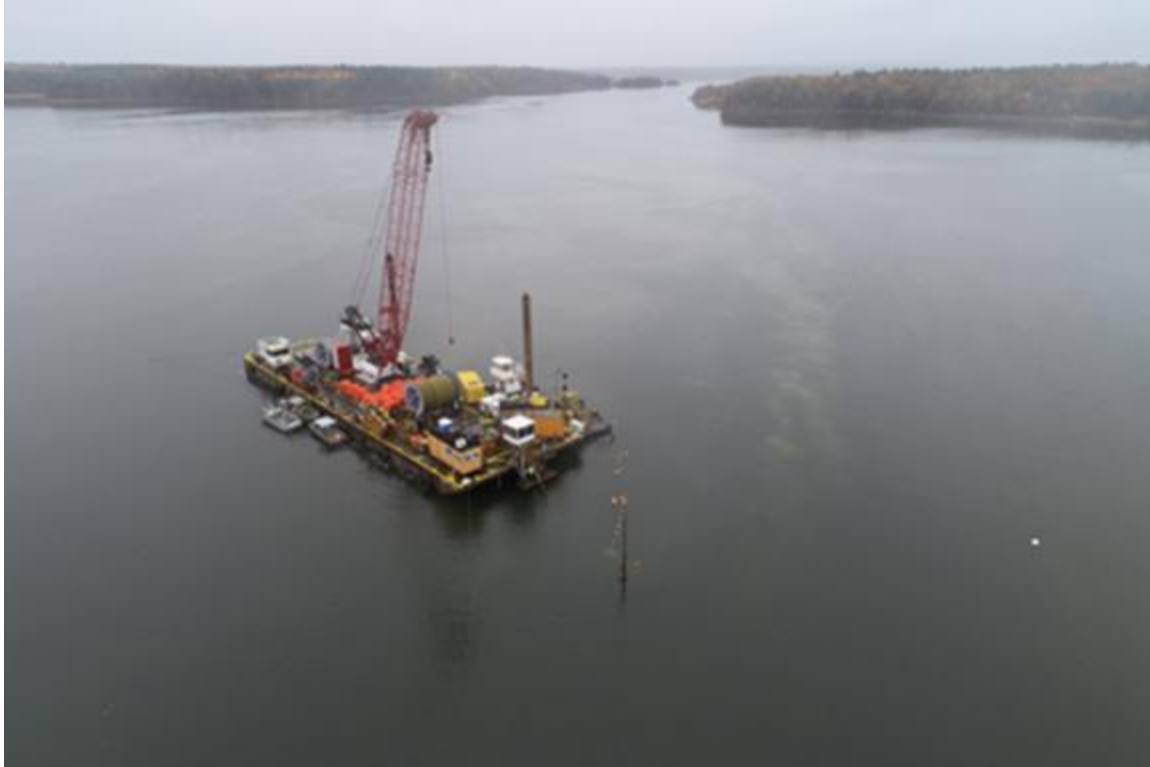
Photo 7. Cable 2, Flight 10, 10/29/2019. Lay barge on channel slope with jet plow behind. Turbidity plume from jet plow is visible on the right.
