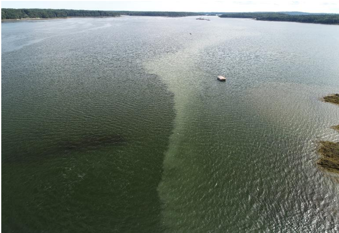
Photo 2. Jet Plow Trial, 9/9/2019. Northern end of turbidity plume facing south from Joe King Oyster Farm. Cable lay barge is visible to the south.
