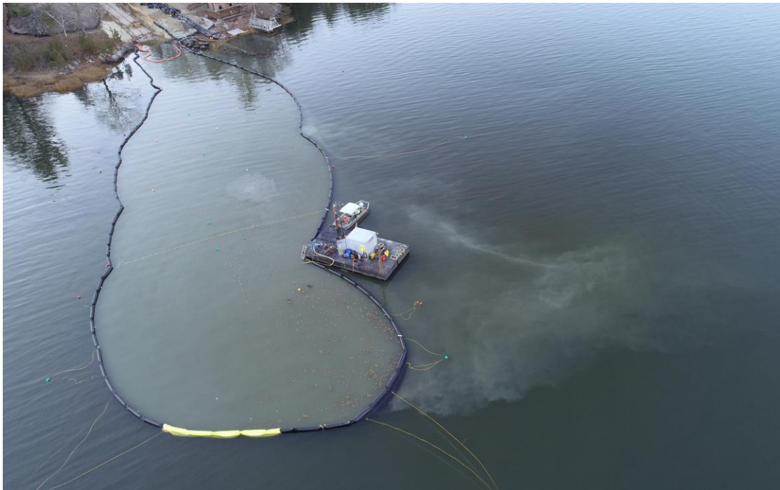
Photo 40. Hand Jet, Flight 1, 11/15/2019. Diver burial inside turbidity barrier on western side on an ebb tide with plume seepage.
