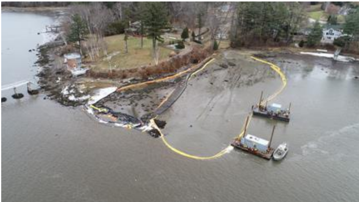
Photo 52. Hand Jet, Flight 1, 12/16/19. Type 1 turbidity curtain installed after turbidity barrier failed on east side.
