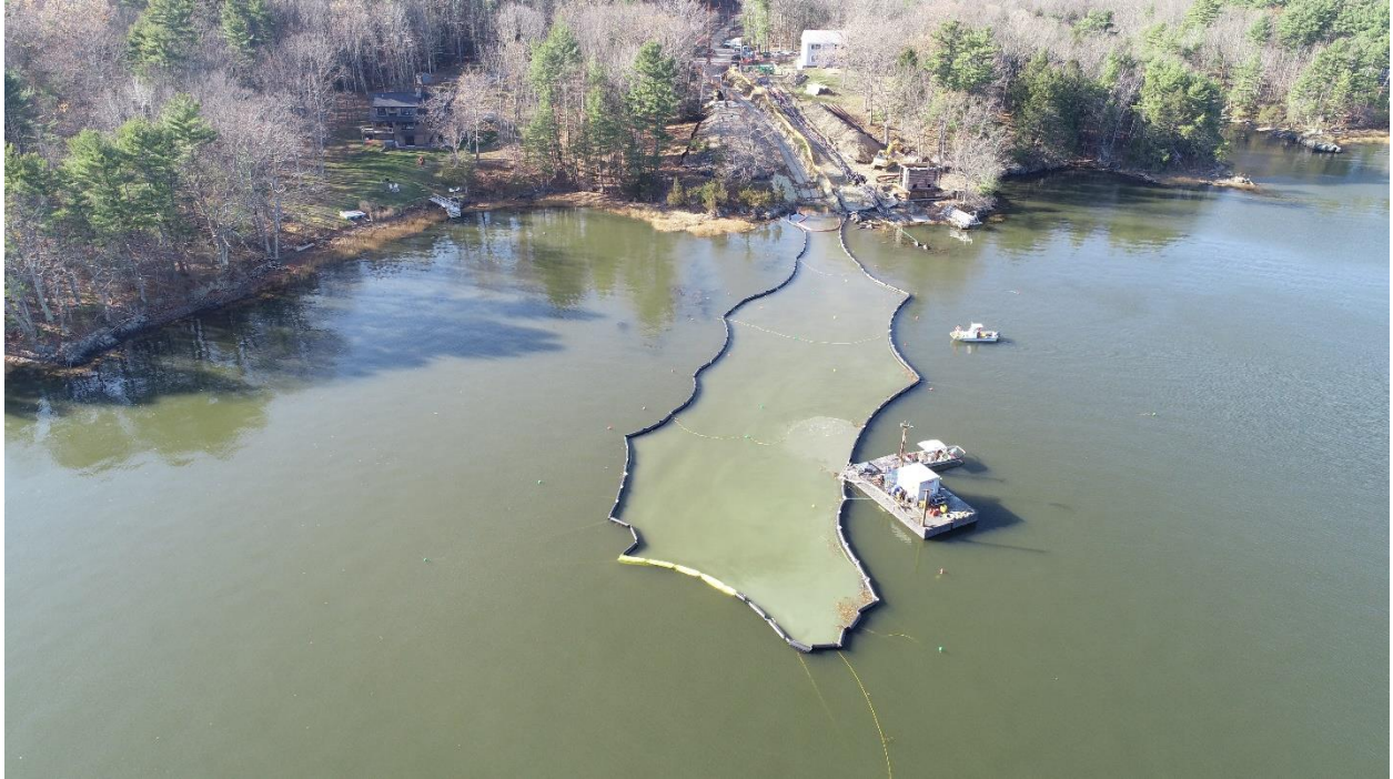
Photo 39. Hand Jet, Flight 1, 11/15/2019. Diver working inside turbidity barrier on a flood tide on west side.
