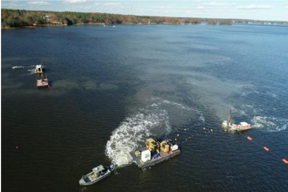
Photo 17. Cable 3, Flight 9, 11/06/2019. Laying cable on tidal flats. At peak ebb, one or more work boats were required to hold jet plow and cable on course.
