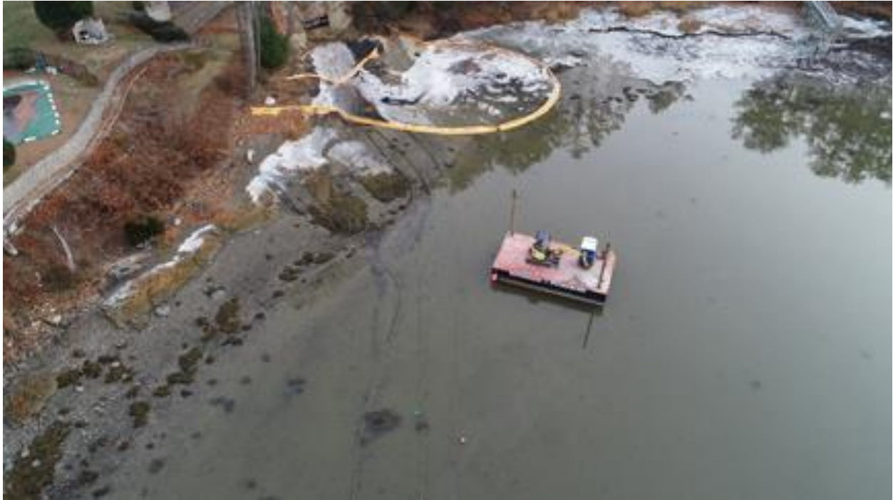
Photo 35. Hand Jet, Flight 1, 11/14/2019. Cables running ashore before diver burial on east side of Little Bay.
