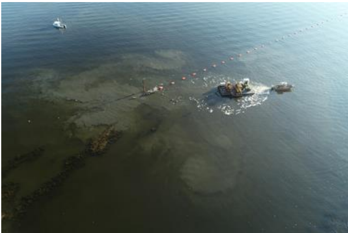
Photo 10. Cable 3, Flight 1, 11/06/2019. Jet plow start on western tidal flat, with pump barge, work skiff and water quality sampling boat at top of photo. Note cable supported by orange floats leading to laybarge.
