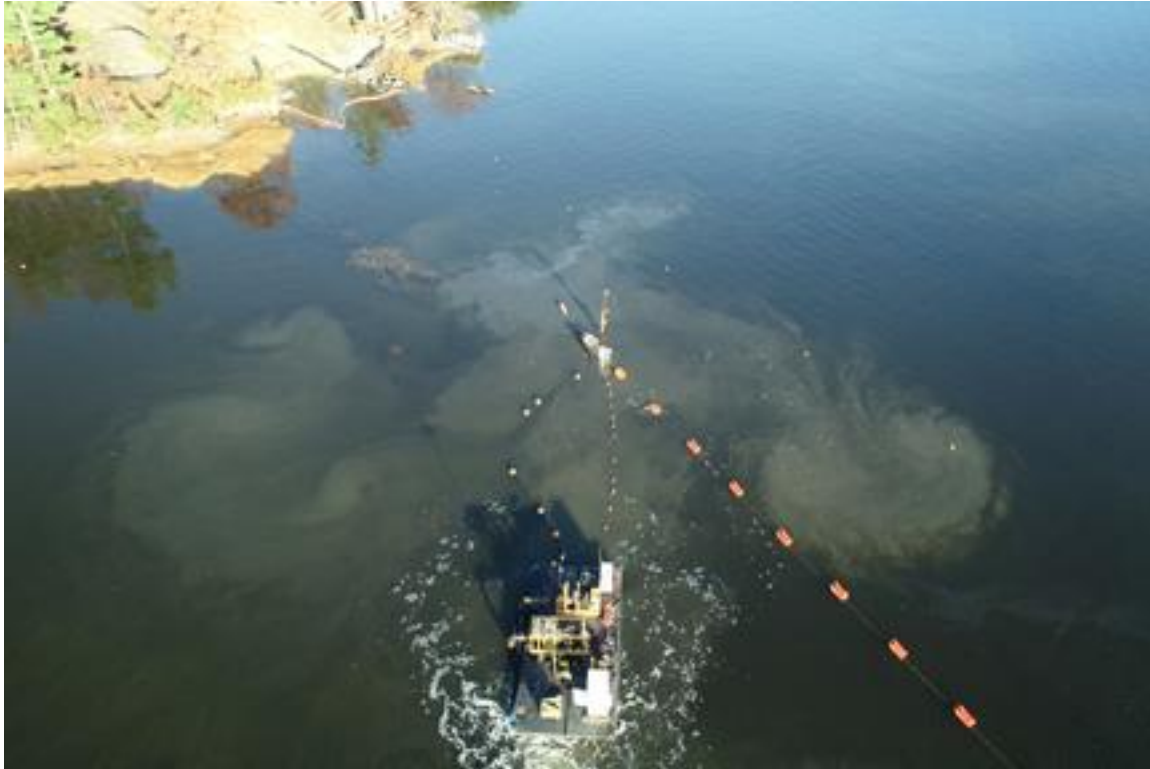
Photo 9. Cable 3, Flight 1, 11/06/2019. Starting of jet plow on western tidal flat with pump barge being held in position by work skiff (not in photo). Note orange floats supporting cable. High slack tide.
