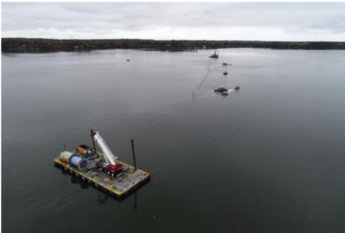
Photo 4. Cable 2, Flight 5, 10/28/2019. Looking east across western flats, showing tender barge, jet plow with attendant work boats, cable on orange floats, and cable lay barge at edge of channel in distance.
