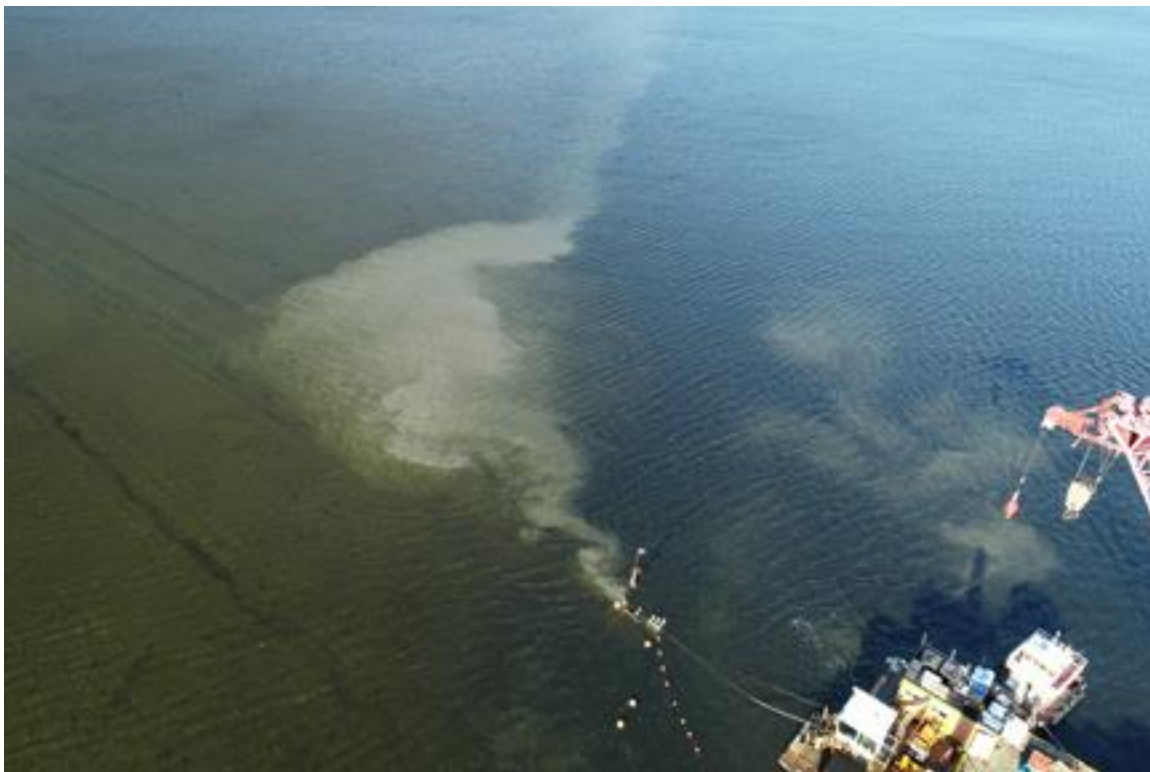
Photo 20. Cable 3, Flight 12, 11/06/2019. Jet plow approaching barge at end of crossing of western tidal flat. Note cable burial tracks on flats.
