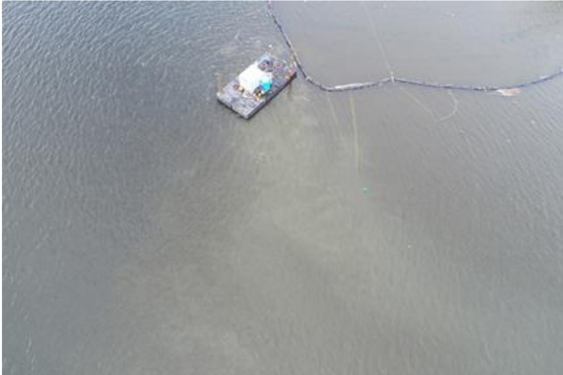
Photo 43. Hand Jet, Flight 8, 12/05/2019. Diver burial for a cable just outside of turbidity barrier on east side.
