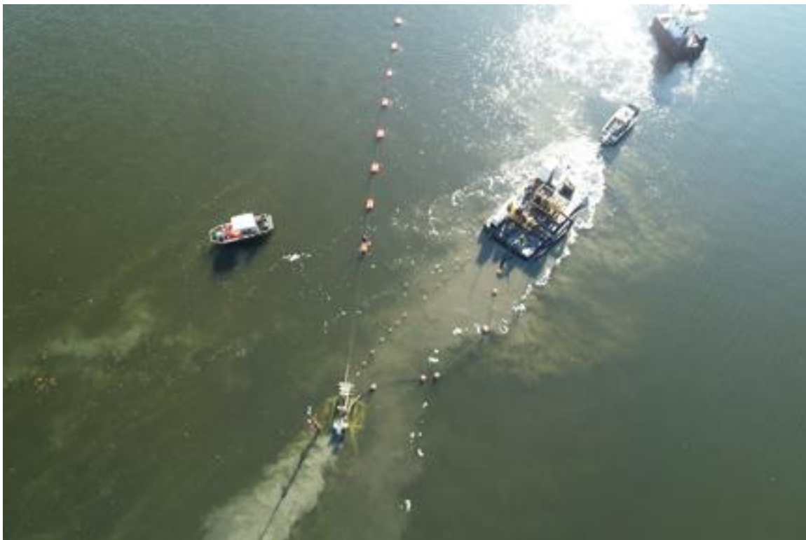
Photo 14. Cable 3, Flight 4, 11/06/2019. Jet plow in lower portion of photo with work skiffs and support barge. Note diver releasing orange floats from cable.
